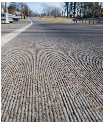
Milled Ductal riding surface on a bridge deck, one year after installation
