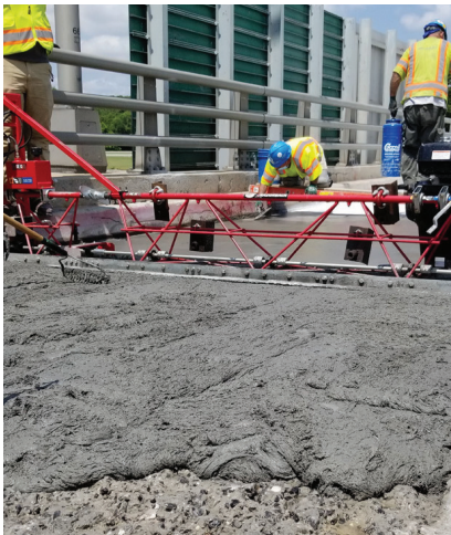
Ductal thixotropic material placed on a bridge deck with a vibratory truss screed
